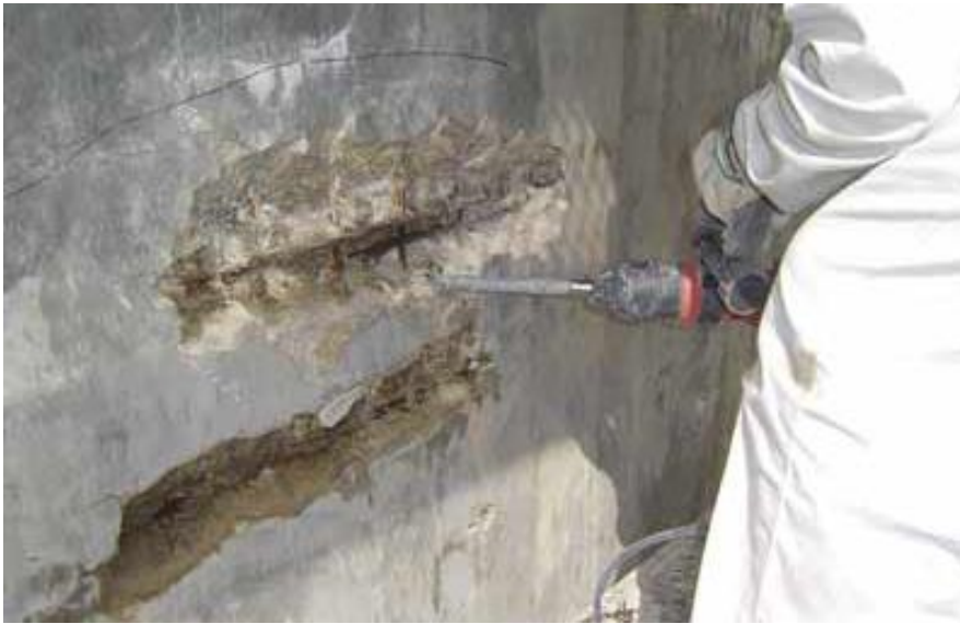
Figure 11. Concrete damage from acids
